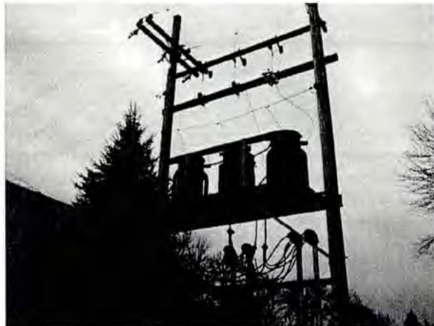
Picture #5: Main Overhead Service
