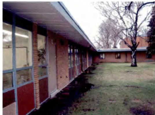
Stanford Centre West Wing. Note ponding of rain water near building and poor site drainage.
