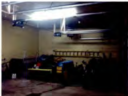
Picture #1: Existing Garage Unit heater and combustion air intake
