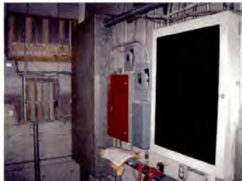
Picture #7: West Wing Electrical Distribution Panel
