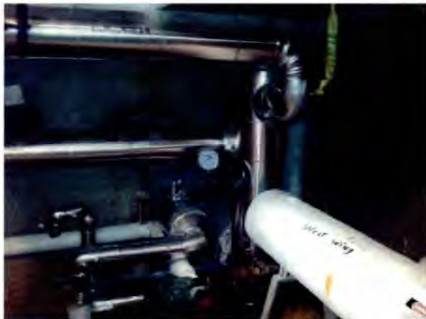
Picture #4: New Steam Piping in the basement mechanical room
