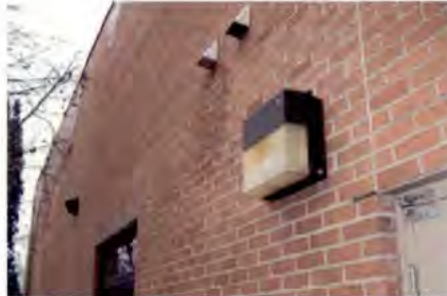
Picture #6: Exterior Lights
