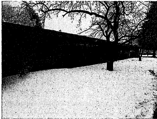
Stanford Centre West Wing showing existing, original window wall system recommended for replacement.
