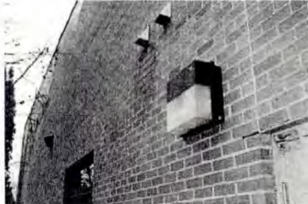
Picture #6: Exterior Lights
