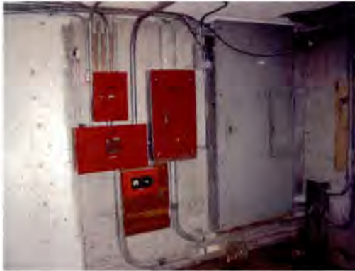
Picture #8: South Wing Distribution Panels
