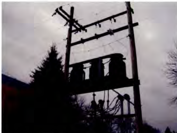
Picture #5: Main Overhead Service
