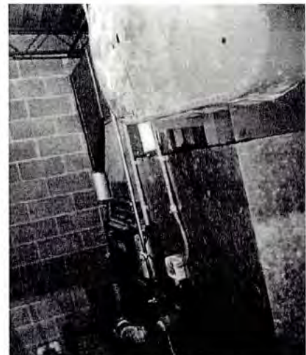
Picture #3: Existing Gym AHU that is not functional
