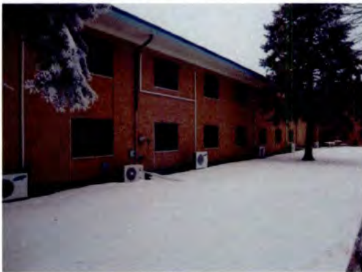
NDVS/SB South Wing. Note multiple split-system air conditioning units. Recommend replacement with centralized system.
