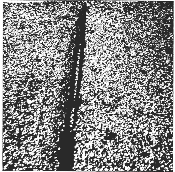
9-16-97 Bisek Hall roof areas A & B expansion joints are split open with air pockets. ----Built 1974
