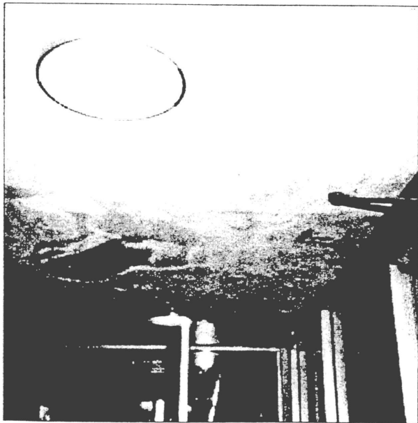
11-5-97 Satterlee Hall roof Area B, water is running through ceiling and wood is getting wet. Wood decking is rotten. ----Built 1964
