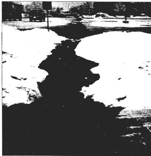
1-30-98 Deteriorated steam lines 14th Ave. to College Complexes.
