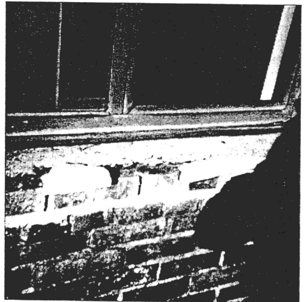
10-28-97 Horton Hall mortar joints and sills are falling off building. ----Built 1927
