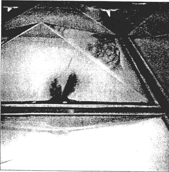
11-5-97 Student Center skylights are cracked and full of water. ----Installed 1968
