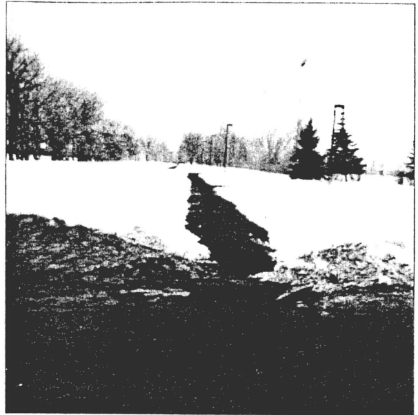
1-30-98 Deteriorated steam lines Blikre Activities Center south to Patterson Maintenance Center.
