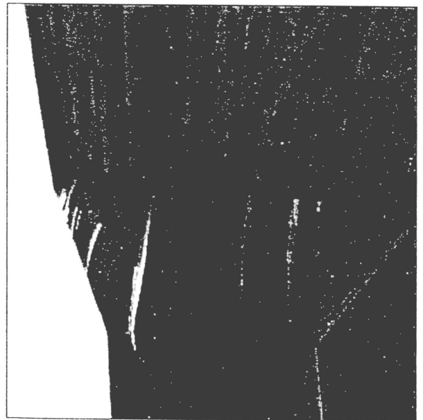
11-5-97 Satterlee Hall roof Area B, water is running through ceiling and wood is getting wet. Wood decking is rotten. ----Built 1964
