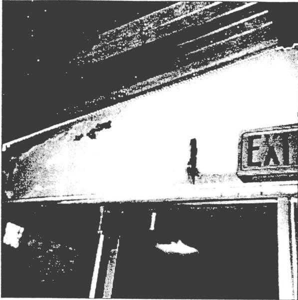
11-6-97 Satterlee Hall roof Area B, walls are rotting from water coming through roof. Lounge area plaster is deteriorating. ----Built 1964
