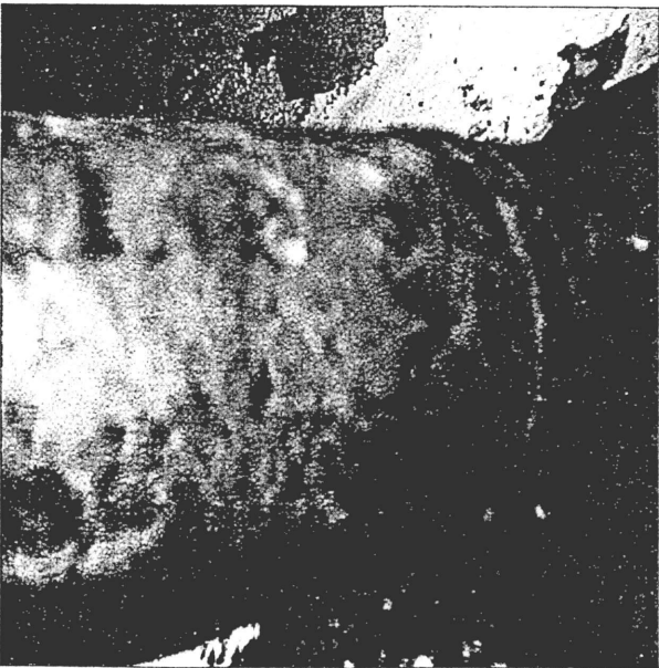
9-16-97 Underground steam pipe south end of campus.
