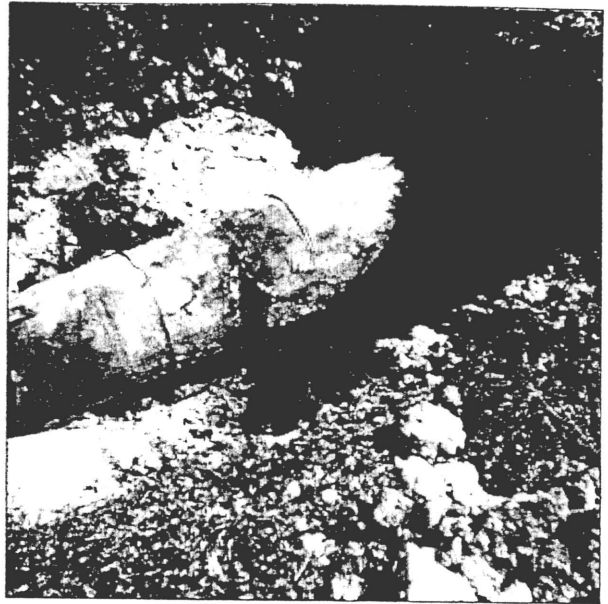
9-17-97 Piping is deteriorated in underground steam lines north end of campus.
