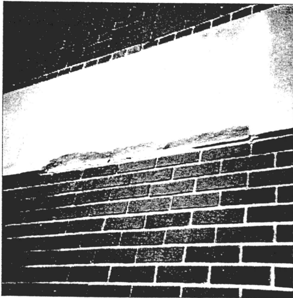
10-28-97 Barnard Hall concrete is cracking and falling off of the building. ----Built 1967
