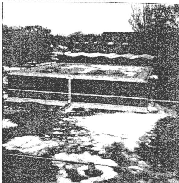
11-5-97 Student Center roof area A-1979, D4-1976 and E-1976. All areas have water leaking into insulation & on decking.
