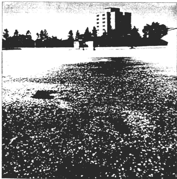
9-16-97 Schuett Hall roof areas B-C-D-E-F-G are leaking in every shop area. ----Built 1976
