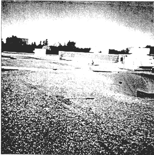
9-16-97 Schuett Hall roof areas B-C-D-E-F-G are leaking in every shop area. ----Built 1976
